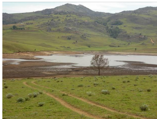
Picture 2: State of Hawane Dam captured during the Deputy Prime Minister's tour of the dam
